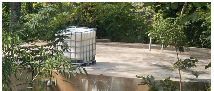
New storage tank on Likwenu River
