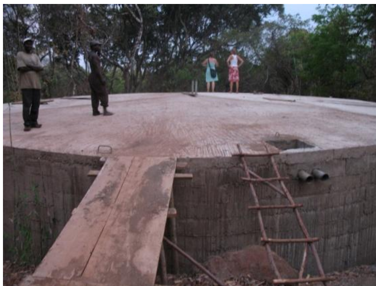
New sedimentation tank
